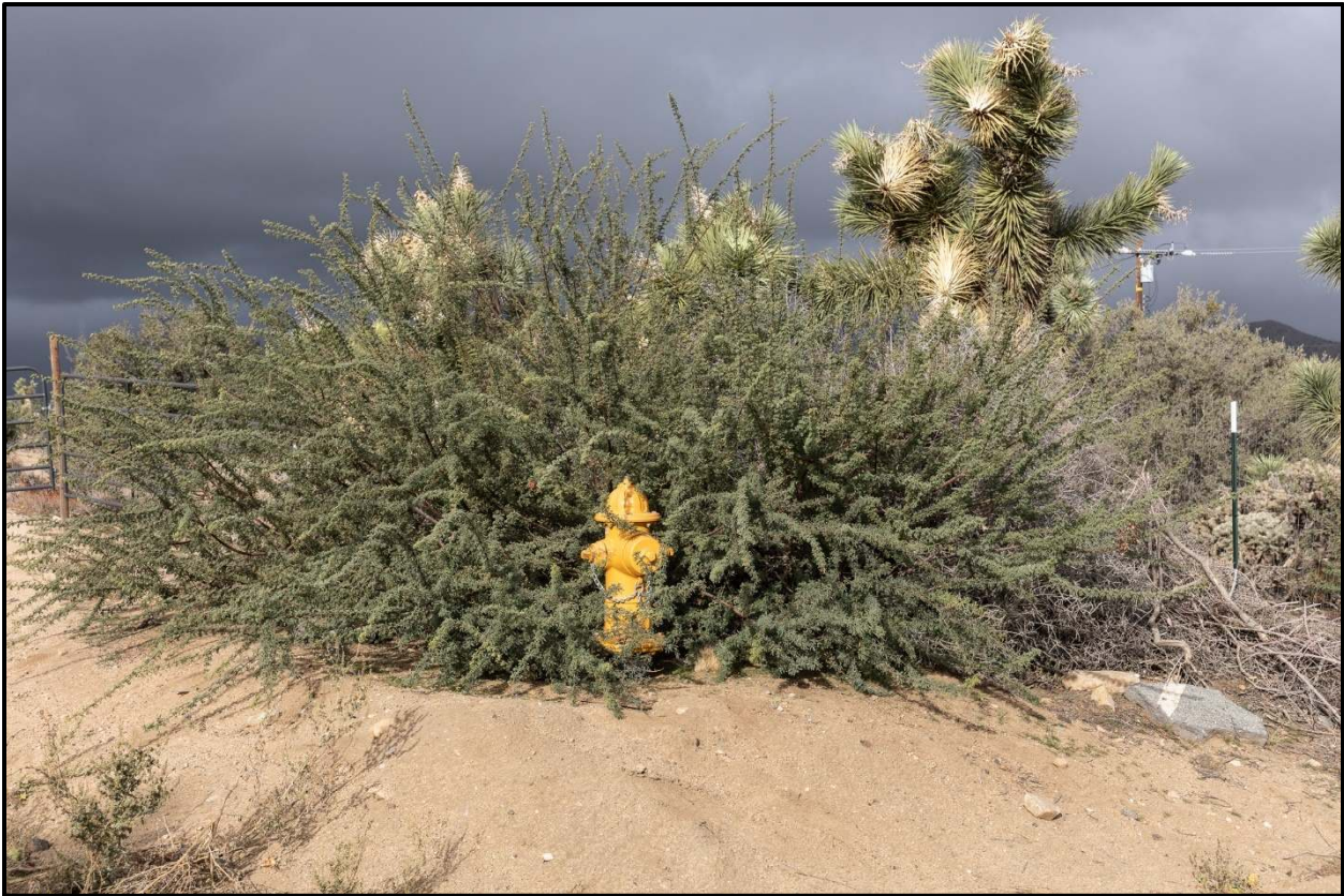
Figure 7, Hydrant Overgrown by Vegetation in Yucca Valley
